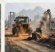
Dust from Construction & Roads
